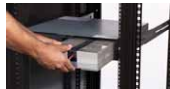
The batteries on this Eaton 9130 UPS are hot swappable.
